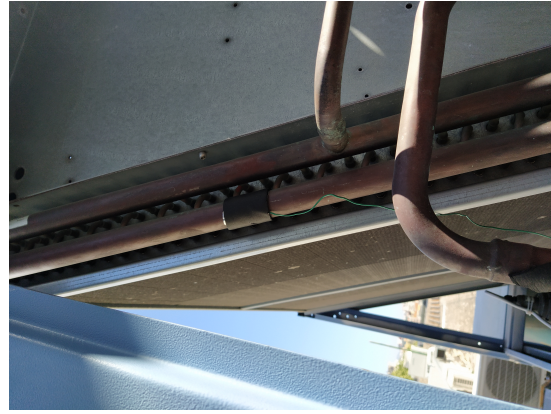
Figure 3.19: Thermocouple applied to condenser coil, and insulating tape on top of it.
